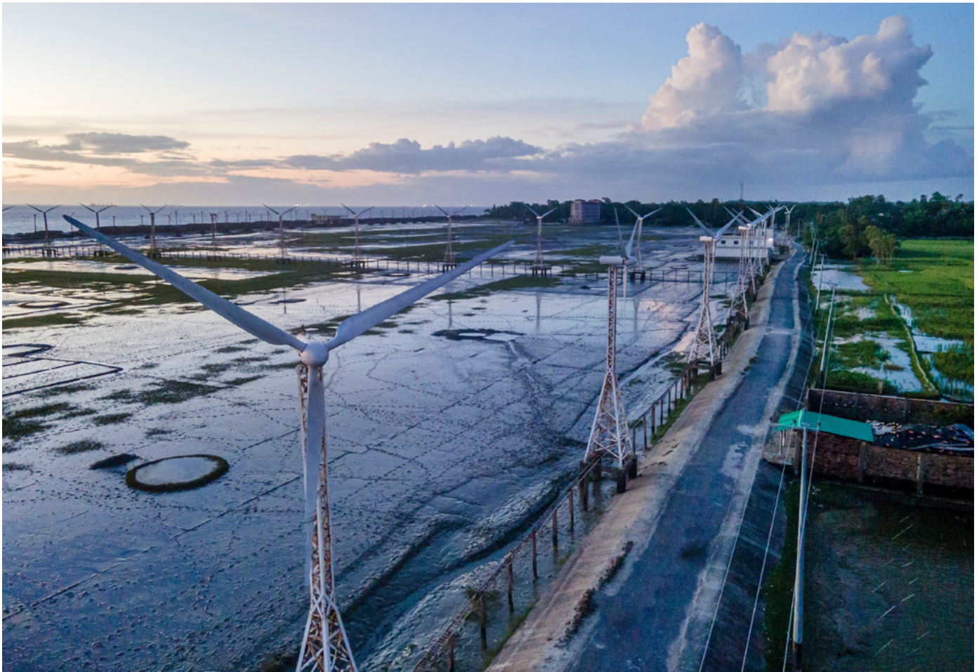
View of the wind power plant of Kutubdia, Bangladesh.
